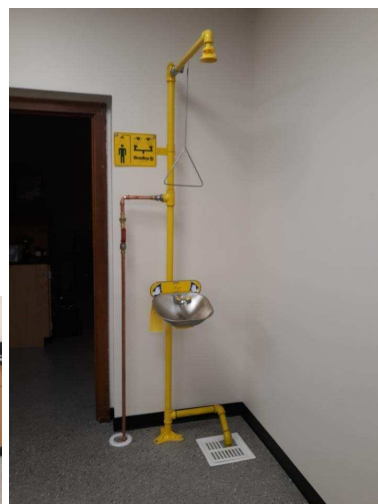
Eyewash/Shower Safety Station
